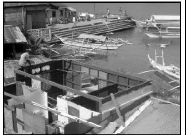
A house missing a roof in Muelle
