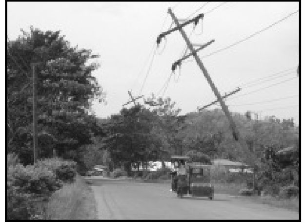
Electric poles atilt perilously at Balatero road
